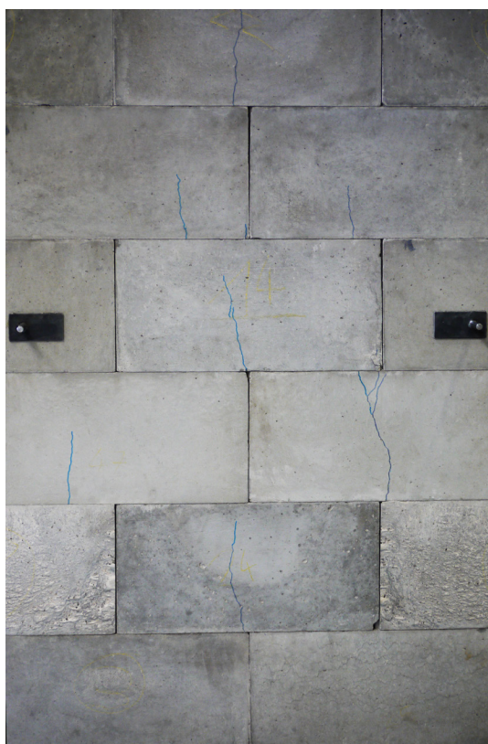
_Fig. 18: Characteristic crack patterns observed during experimental investigations involving vertical loadings and bending moments on stretcher-bonded and dry-stacked masonry structures
